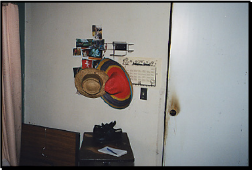
Figure 7 - Interior of patient room, where the door was closed during the fire (NFPA)
